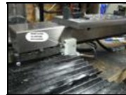
X Axis Limit Switch Covered
