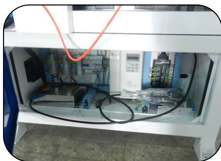
Electrical Control box
